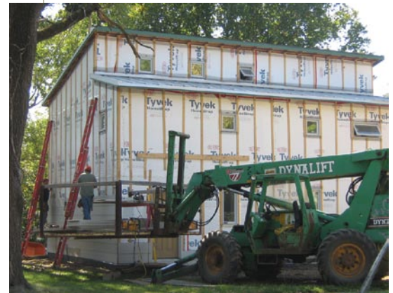
The Fairview house—shown during and after construction—features 14-inch walls with high-density blown-in fiberglass.
