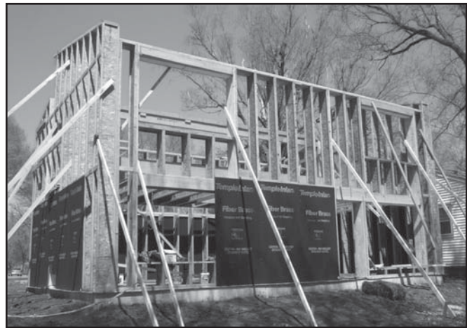
Figure 3. The Passivhaus walls were framed with 14-inch TJIs and sheathed with 1/2-inch asphalt-impregnated fiberboard.
